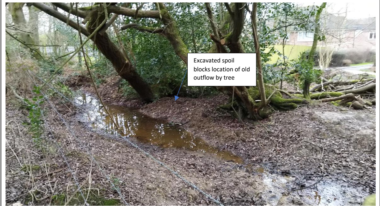
Figure 15, Ditch February 2022. Outflow by Tree Blocked.
