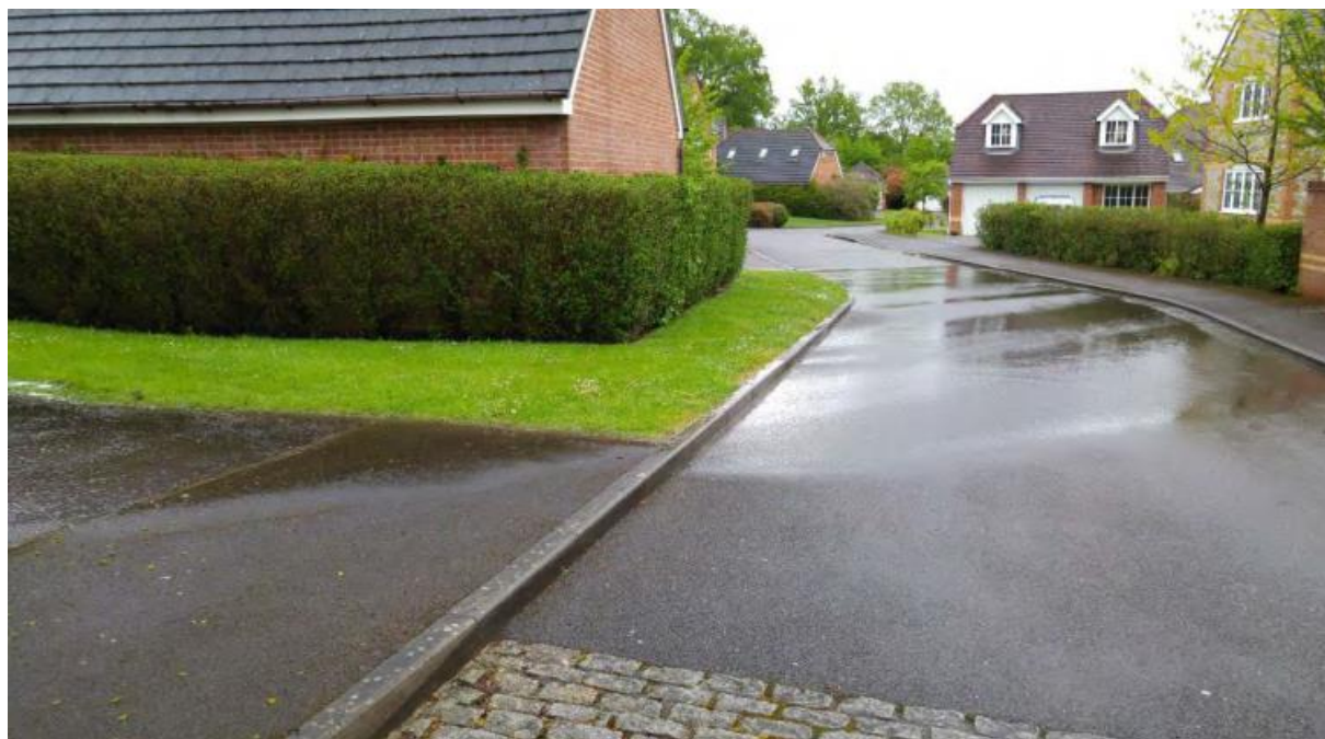
Figure 18, Water Flowing from Access Path and Across the Hardtop, 2016 from John Leeson
